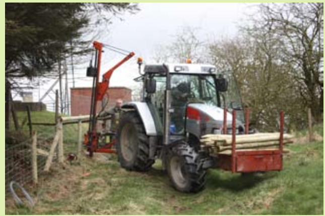
■ Fencing in progress on the northern side of the monument. The fencing was carried out as part of the original purchase agreement with Leighton Estates and was carried out with Scheduled Monument Consent. Photo CPAT 2830-0017.
