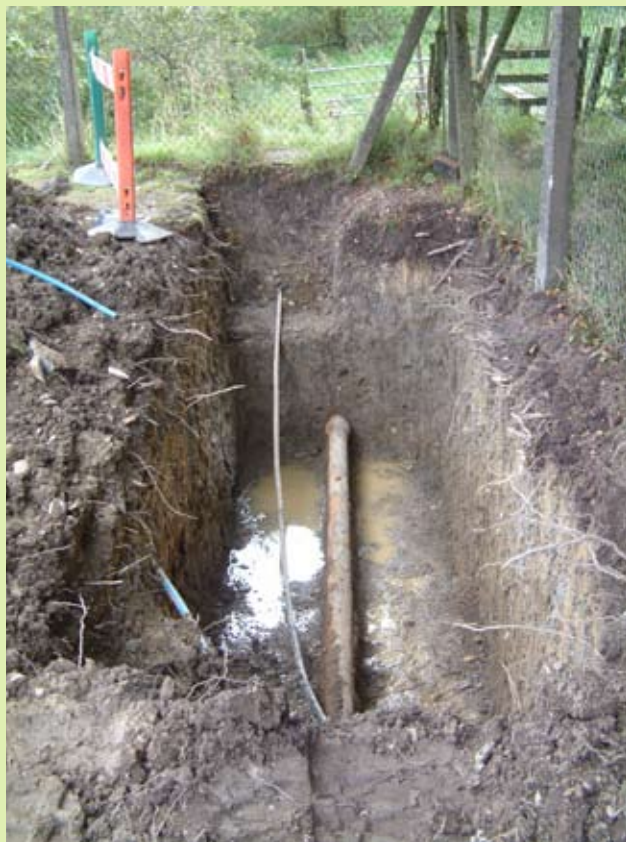
■ Work by Severn Trent Water in the compound just to the north of the site showed the depth of natural clay which caps the top of Long Mountain at this point. Photo CPAT 2641-0011
